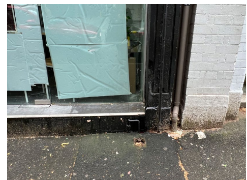
Figure 4-8: Street level and internal floor level at 244 Reservoir Street (former 242) (Source: Curio 2022)
