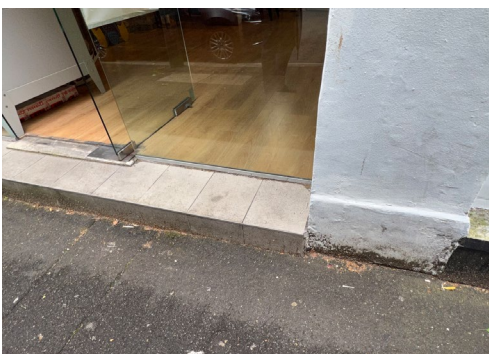
Figure 4-7: Street level and internal floor level at 242 Reservoir Street (former 240) (Source: Curio 2022)
